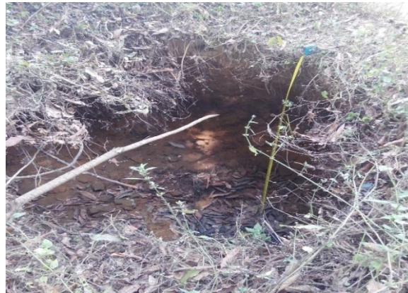
Plate 2: Sinkhole at Ediganang
